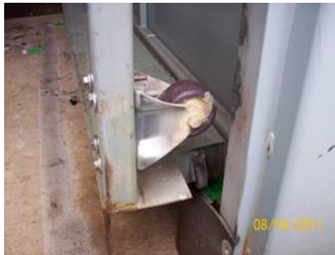
Damage to lower part of baggage lift cradle
