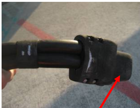
Damage to GPU cable power plug
